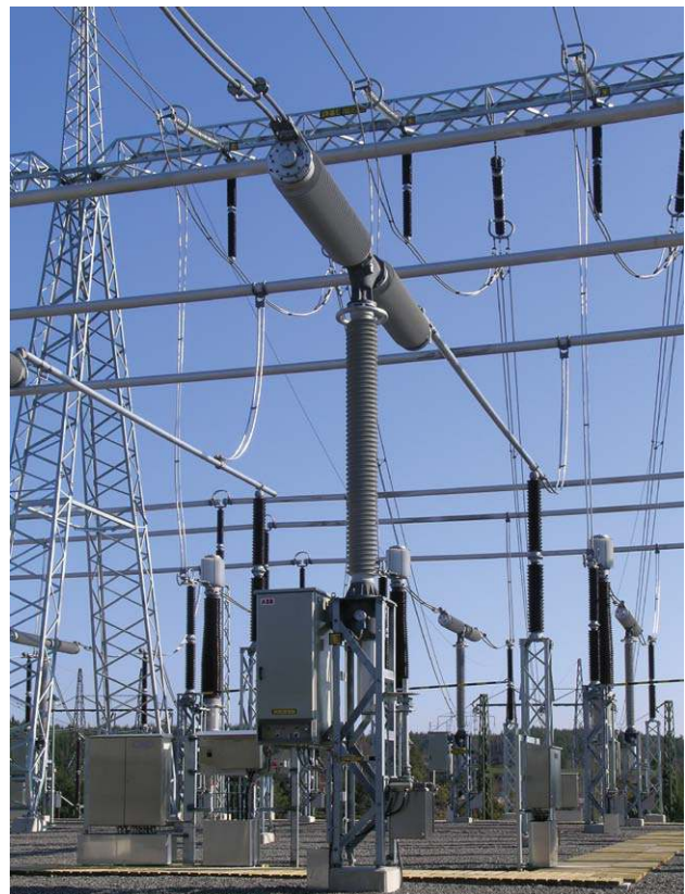
HV Transmission circuit breaker
