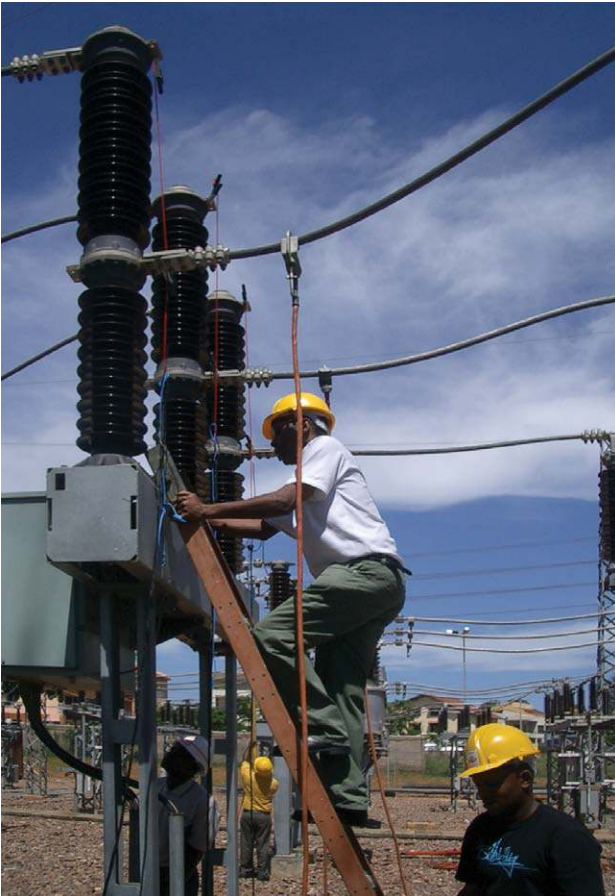
Circuit breaker grounded during preparation for timing test
