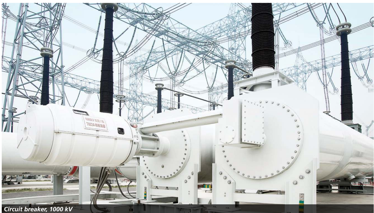
Examples of bulk oil circuit breakers
