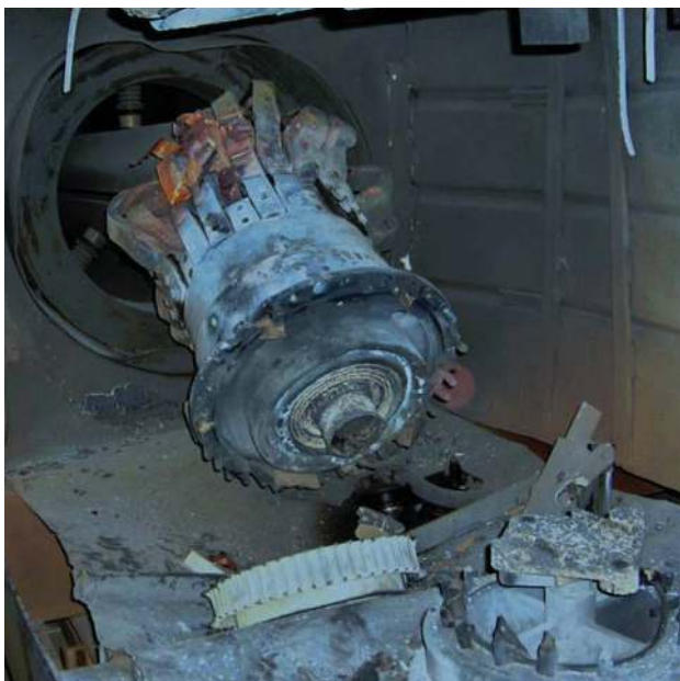
Generator circuit breaker failure
