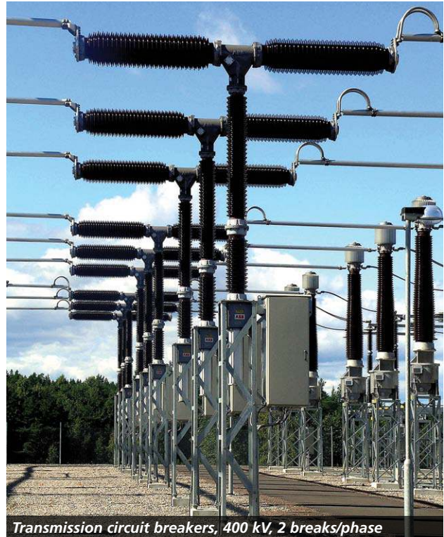
Transmission circuit breakers, 400 kV, 2 breaks/phase
