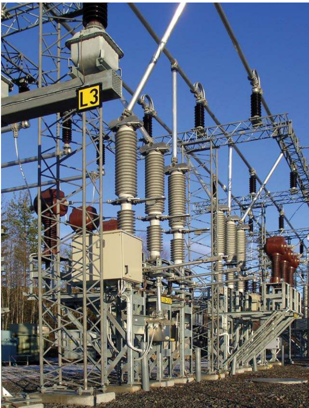
72 kV Distribution circuit breaker
