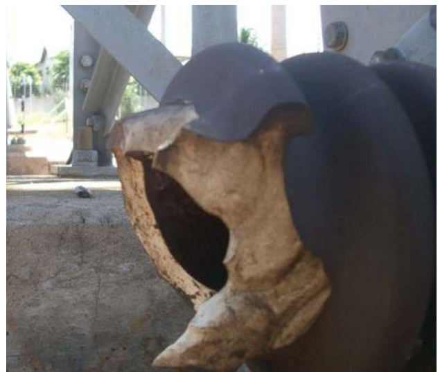
A distribution circuit breaker pole totally damaged by explosion.
