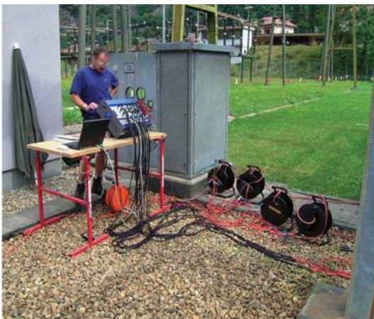
Circuit breaker hooked up for test and measurement.
