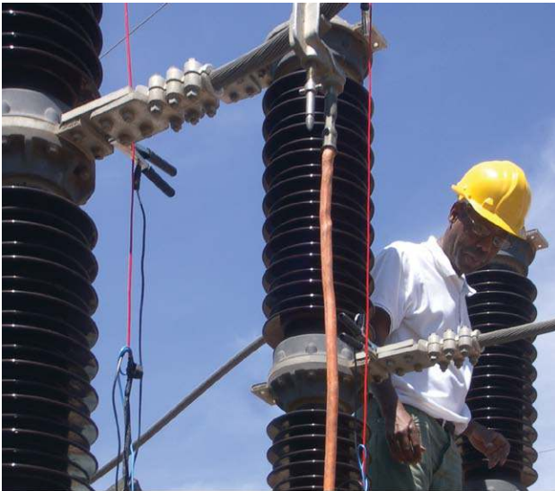
Connection of cables and clamps on a distribution CB.
