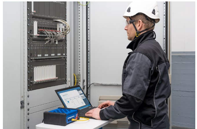
Figure 3: StationGuard imports the SCL (Substation Configuration Language) file of the substation to create a complete system model.
