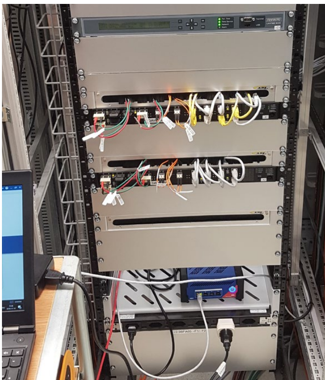
Figure 4: Pilot installation at a 110kV substation of CKW.
